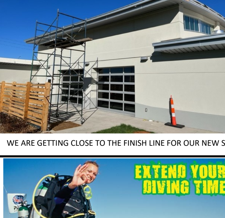
WE ARE GETTING CLOSE TO THE FINISH LINE FOR OUR NEW SCUBA AND SWIM HEADQUARTERS. STAY TUNED FOR MORE NEWS!
